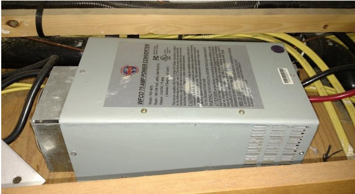
RV power converter
